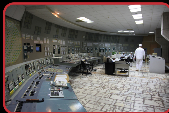
Figure 27 Control Room of Chernobyl Nuclear Power Plant
